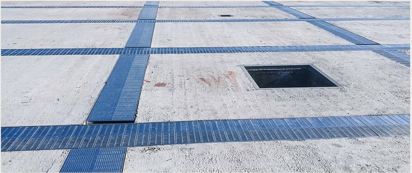
Aeration channels and grids. Photograph: AGI.
